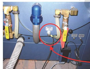
Ground Wire Connected to Chamber
